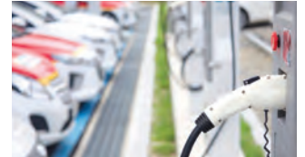
Electric Car Charging Stations
