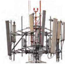
Remote Radio Units (RRU)
